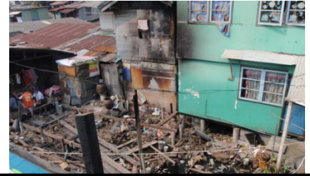
Fire damage area near Day Care
